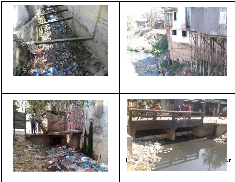
Drainage congestion due to uncontrolled dumping of solid wastes in Sylhet, Bangladesh
